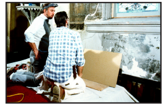
A 1985 photo of artisans discovering the trompe l'oeil art around the windows using controlled paint removal
